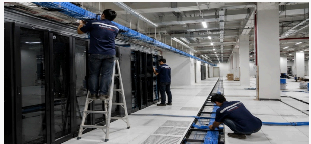
Structured Cabling & LAN Infrastructure
